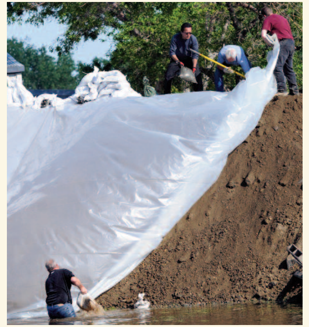
Work proceeds on a dike, privately built to protect a small business.
