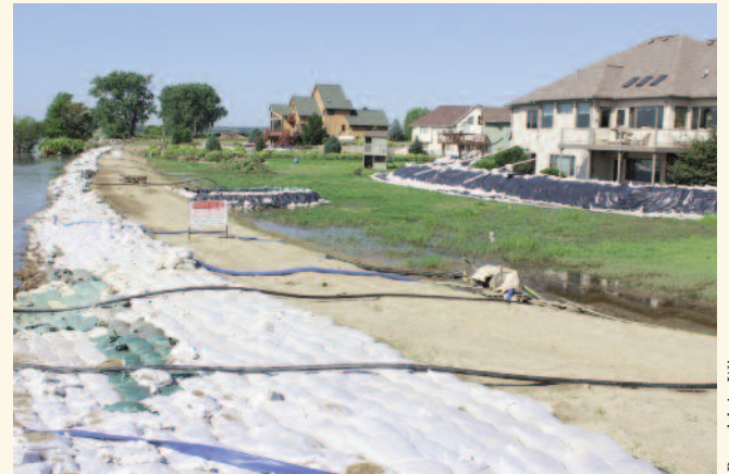
Multiple pump hoses carry groundwater over a dike in rural Union County, S.D.
